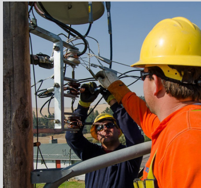
Avista personnel install smart transformers to help improve the efficiency of the Pullman distribution system.
