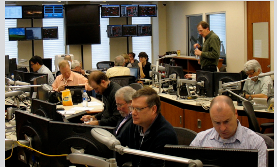
In a step toward establishing the demonstration project's transactive system, in April 2011 engineers from the Bonneville Power Administration and Alstom Grid successfully established a digital data connection to the Electricity Infrastructure Operations Center (EIOC) at Pacific Northwest National Laboratory. A week later, 25 participants from four of the project's technology firms also demonstrated this connection at the EIOC and conducted additional testing.
