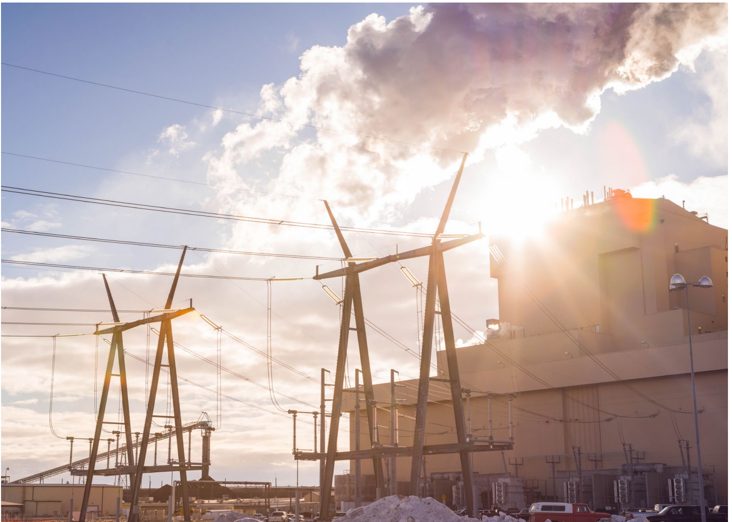
Transmission lines are centered around the Colstrip Power Plant.
