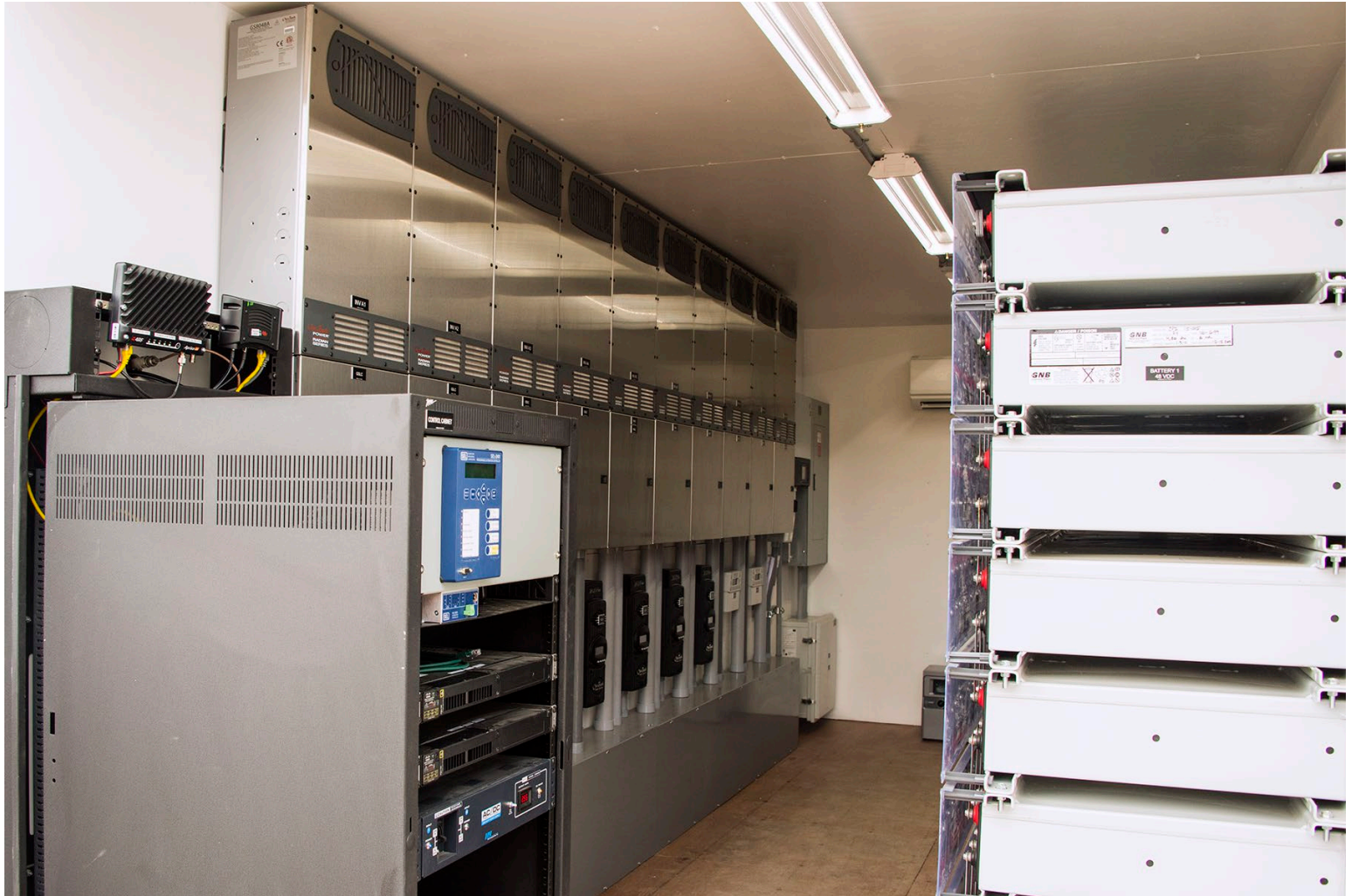
The grid-connected Beck Hill Microgrid pilot project, located near Deer Lodge, Mont. uses an array of ground-mounted photovoltaic panels and inverters to generate electricity when conditions permit. Additionally, a battery bank allows this energy to be stored for use during outages and provide grid support during normal operations.
