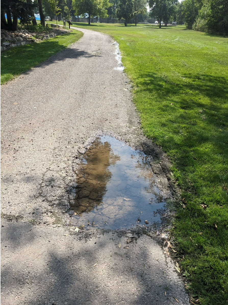
Trail segment surroundings and deteriorated pavement conditions
