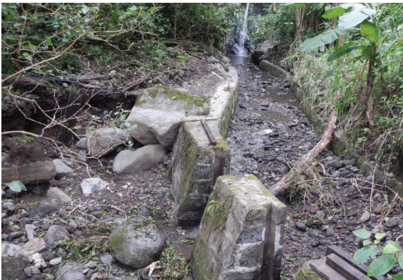
Below Settling Basin Before Cleanout - USDA Photo
