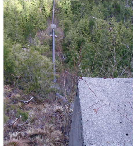
Steep Penstock Drop
