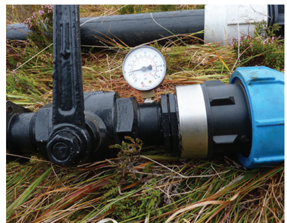
Pressure Gauge Above Turbine Stop Valve
