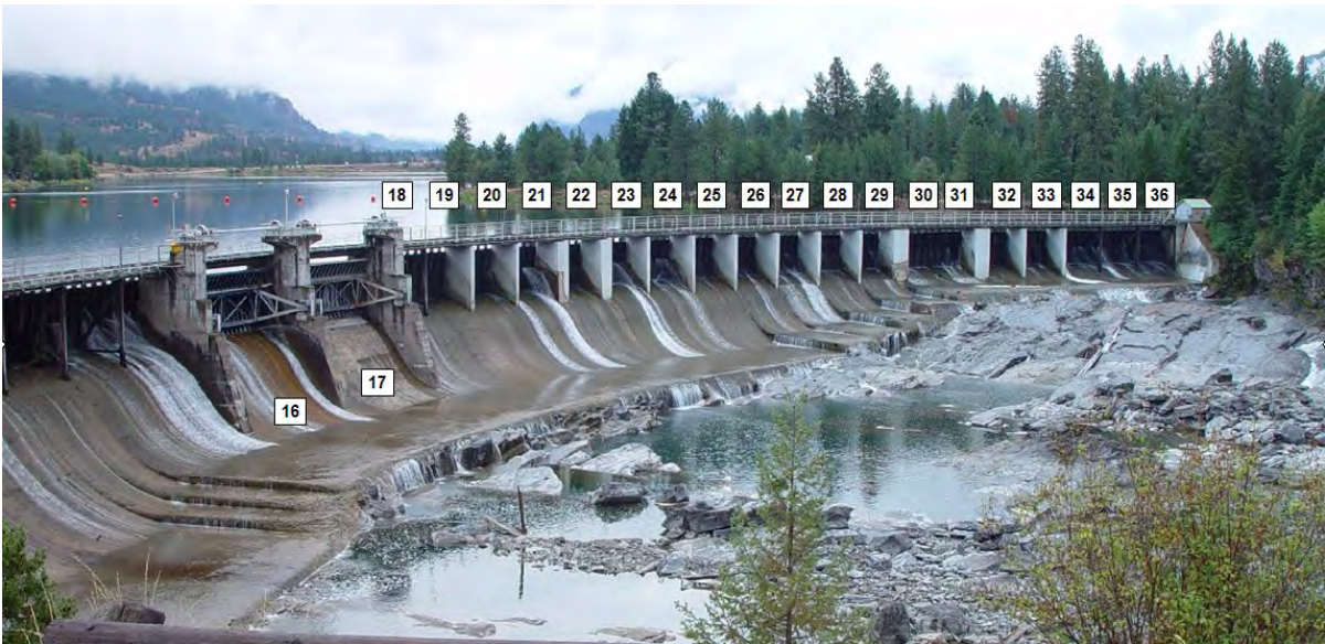
Photo 2. The left bank of the Main Dam at the Thompson Falls Project, with the spillway bays numbered.
