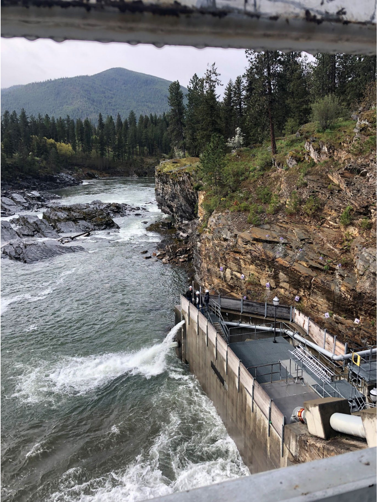
Figure 2-11. Looking Downstream from Main Dam, Upstream Fish Passage Facility on Right, With Auxiliary Water Supply and HVJ
