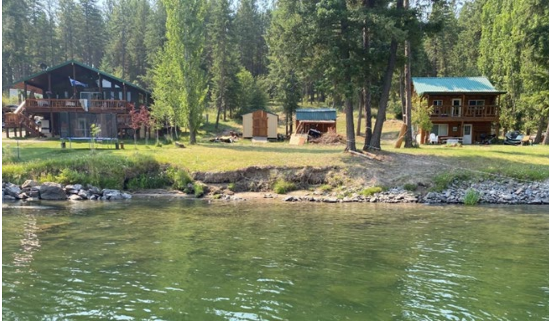
Photo 3-12. Slumped Shoreline – Nick Point Created by the Upstream Rock Rip-rap (left side of photo)
