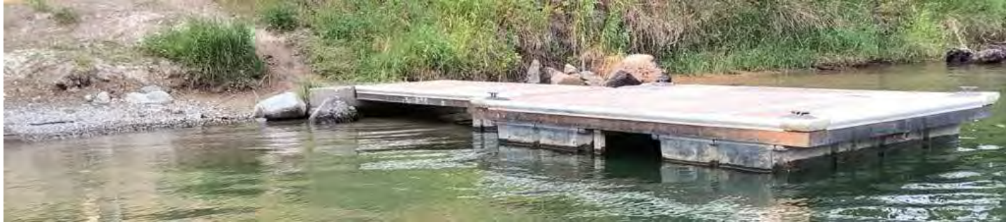
Full Pool Cherry Creek Boat Launch site floating launch dock
