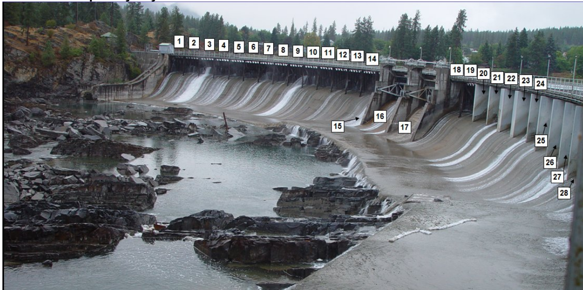
Photo 6-1: The right bank and center bank of the Main Dam at the Thompson Falls Project, with spillway bays numbered.
