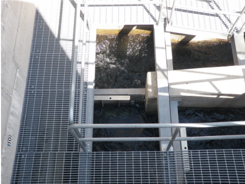
Photo 2: Turning pools 9 (top left) and 10 (lower left). Note increased turbulence in downstream pool.
