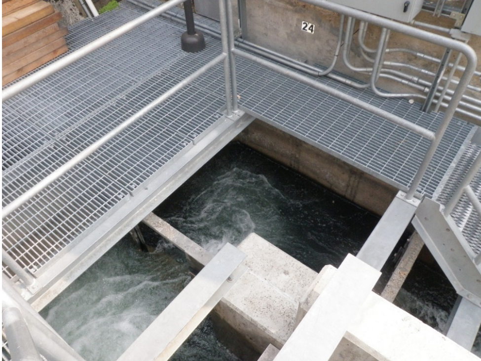
Photo 9: Note difference in turbulence between turning pools 24 (top) and 25. Pool 25 had a plunging nappe, with a depth of flow of 1.34 feet over the upstream weir and no tailwater submergence. Pool 24 had a depth of flow of 0.83 feet over the weir with 0.3 feet of tailwater submergence.
