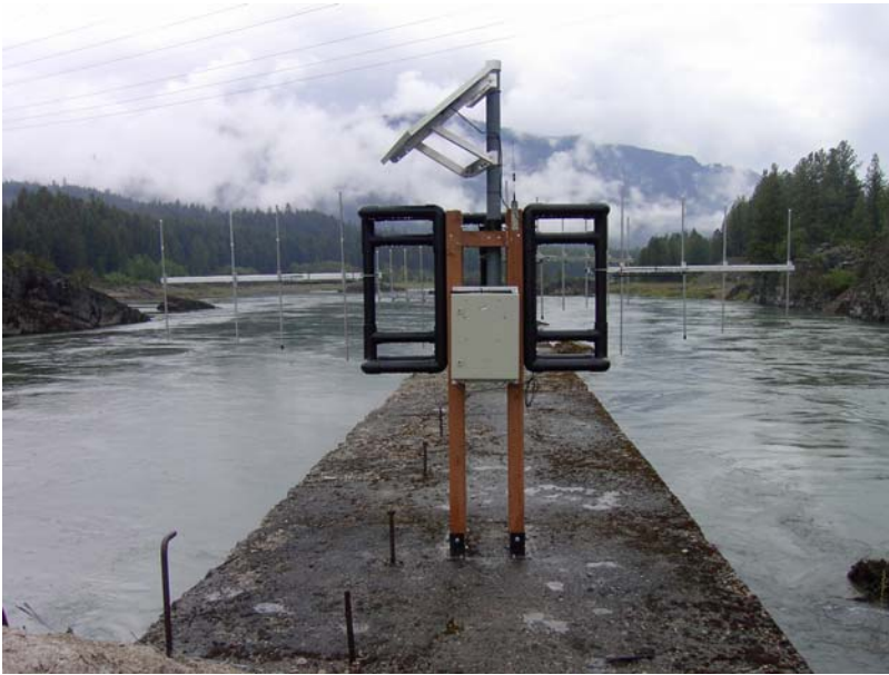
Figure 5: Telemetry monitoring station set up on the wingwall
